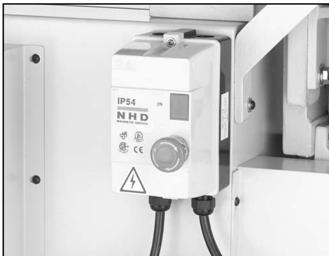
Figure 9. Magnetic power switch.
